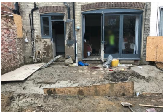
An HSE picture of the accident scene
